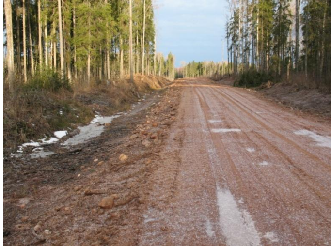
Picture 2. Well drained and bearing road body built of fine soil dug from the ditches and a proper pavement. Tikhvin region, Russia
