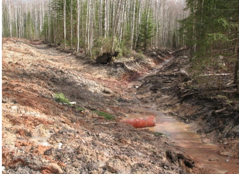
Picture 1. Proper drainage of forest road body on a difficult soil. Tikhvin region, Russia
